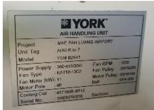
Name Plate AHU
