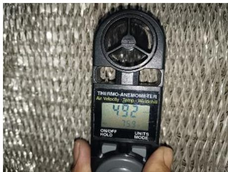
Air Flow with Filter
